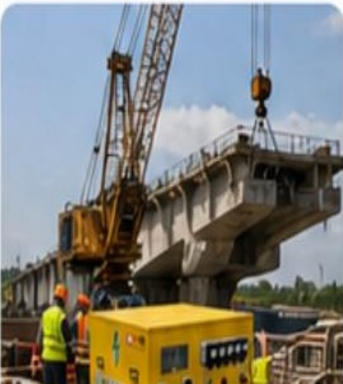
4 Outdoor construction power
