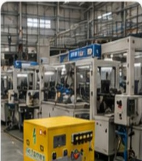
3 Temporary factory power
